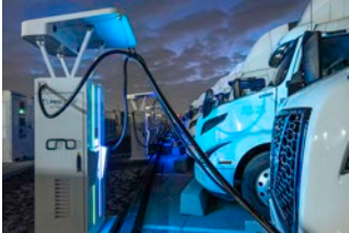
A new electric vehicle (EV) truck charging depot launched
