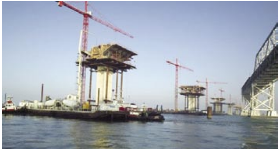
A photo from the Caltrans website shows part of the construction of the new eastern span of the San Francisco-Oakland Bay Bridge next to the current structure.
